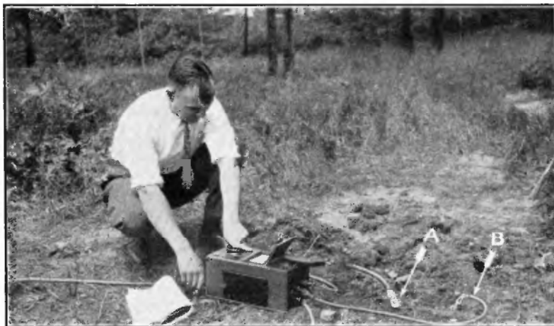
FIG. 9. Testing a substation ground connection with the "Megger" Ground Tester. A is a lead to a portion of the ground network which is disconnected from another portion of the ground network at B . There was so much stray current in the earth around the station that a 100-watt lamp glowed perceptibly in bright sunlight when connected between A and B . The instrument gave consistent results even when A was used as a reference ground.
