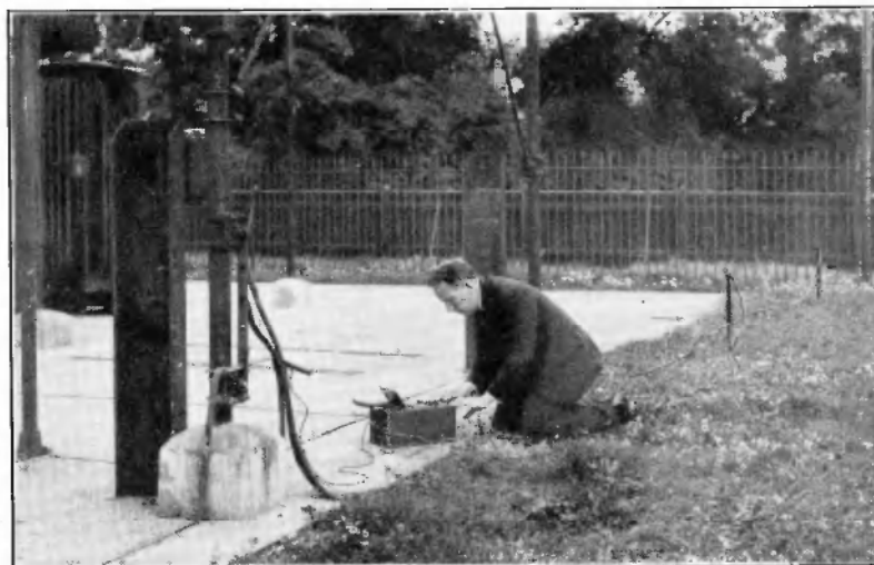
FIG. 30. Testing the resistance to earth of a substation ground connection, using the "Megger" Ground Tester.
