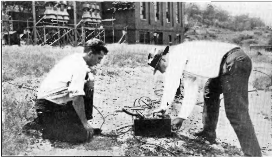
FIG. 18. Testing the resistance to earth of a combined substation ground, which is made up of a large number of separate ground connections,—rods, pipes, steel structure, etc.—tied together.
